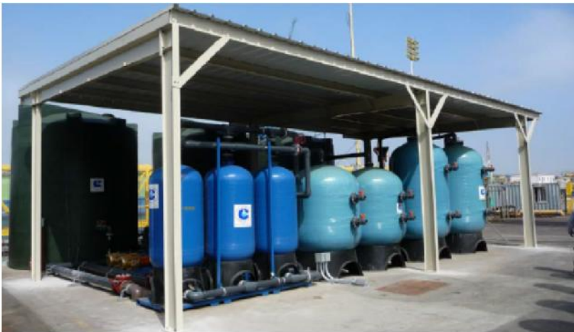
Target Pollutants: Copper, Zinc, Nickel and Cadmium San Diego Industrial Facility Features: 300 GPM Capacity | Discharge to Marine Waters
